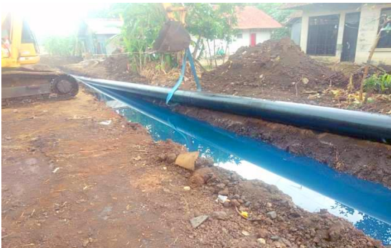
Figure 8 . The leakage of pipes leads to the contamination of the environment and poses a potential risk of fire as it involves the release of oil from the pipes [20]
